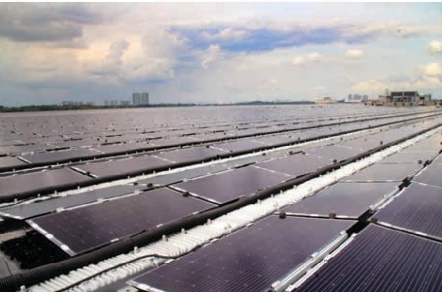
Offshore Floating Solar Farm, Woodlands Senoko
