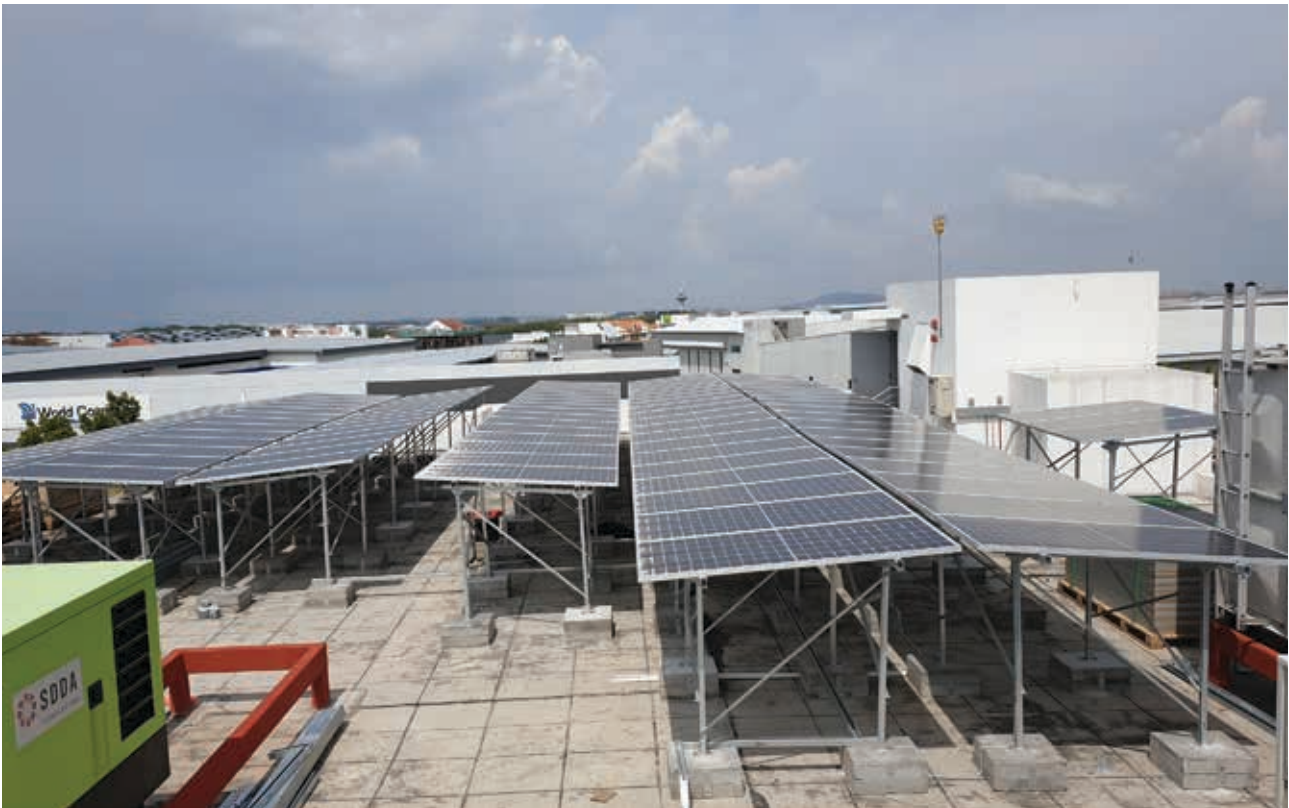
Solar Panels at ISOTeam Headquarters
